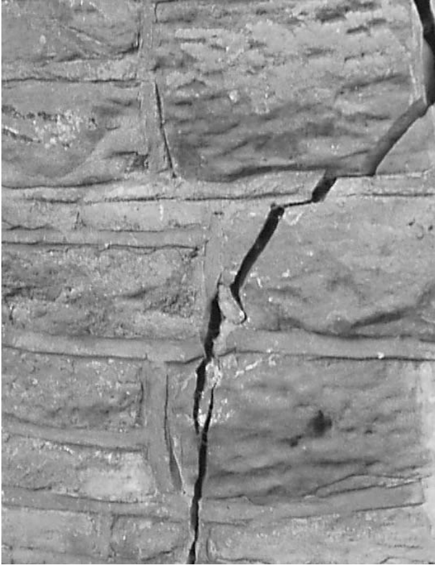
Photo 1: damage after freezing following pointing with Portland Cement Mortar
