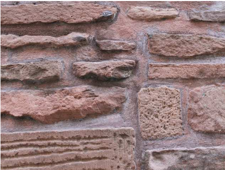
Photo 2: pointing slightly recessed with surface of stone.
