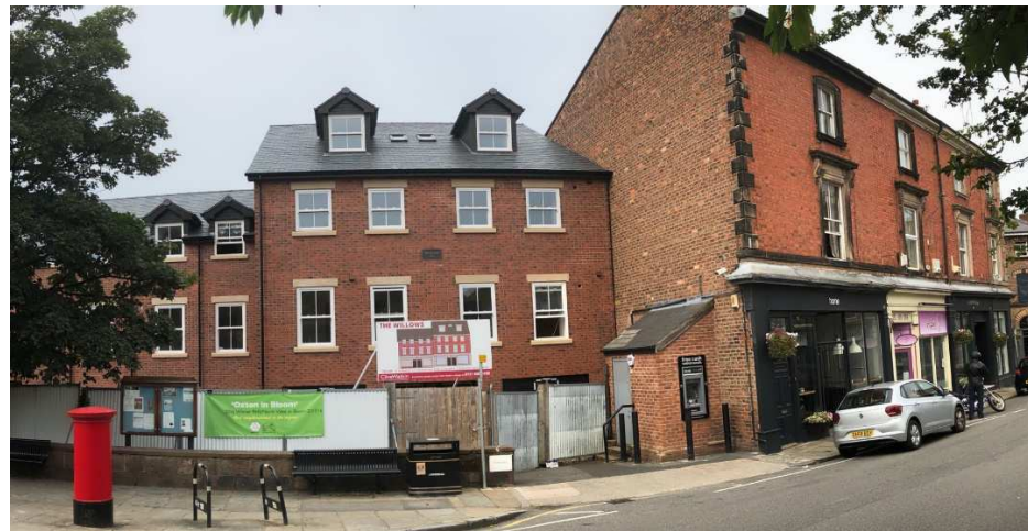
Fig. 33 “The Willows” is nearly completed but just needs the fence removed and the front of the development landscaped
